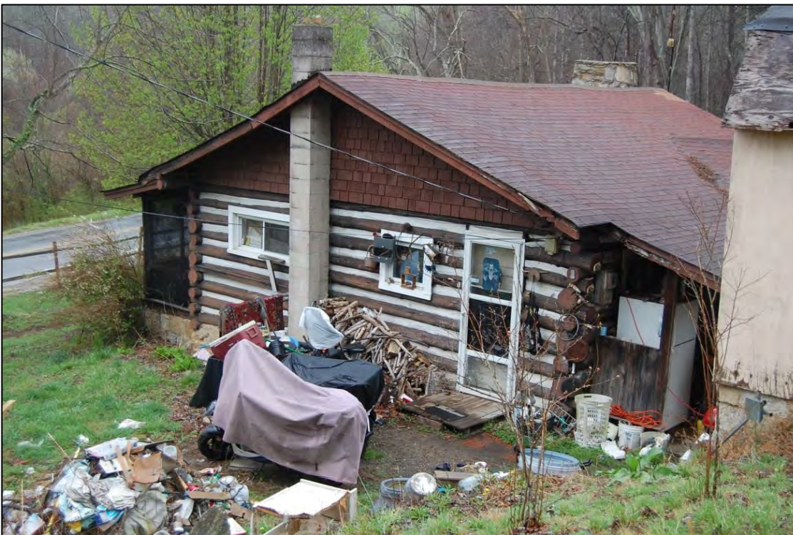
Figure 80. South side and east rear elevations of house; gambrel-roofed shed at right
