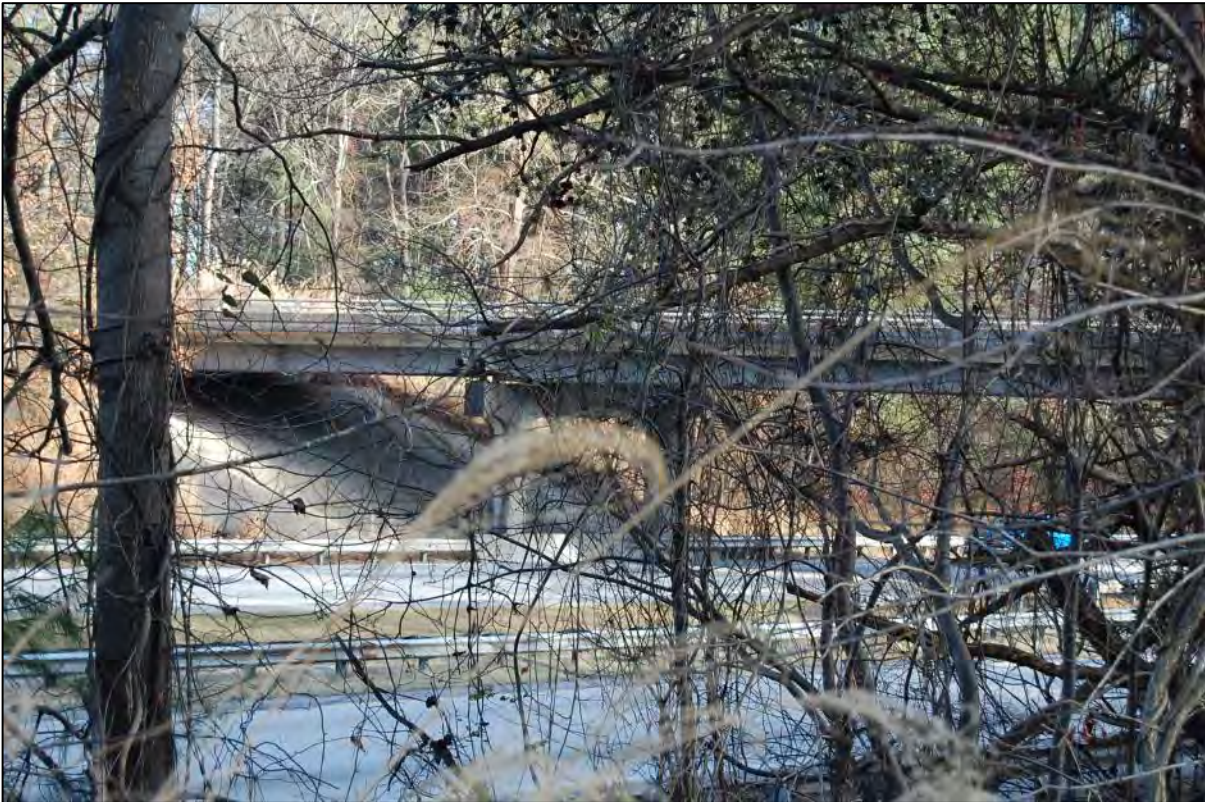
AECOM #47 (HN1963) - Clear Creek Rd over I-26: view looking E at bridge
