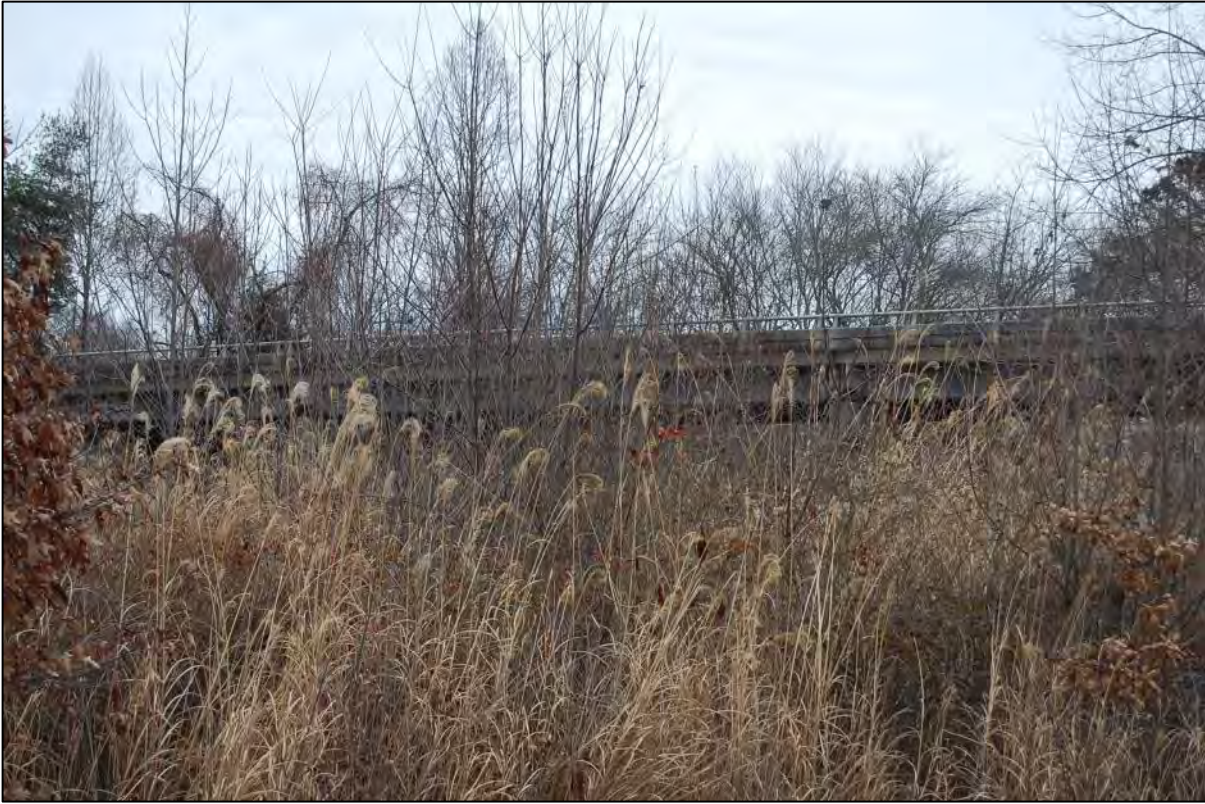
AECOM #44 (HN1964) - Brookside Camp Rd over I-26: view looking E at bridge
