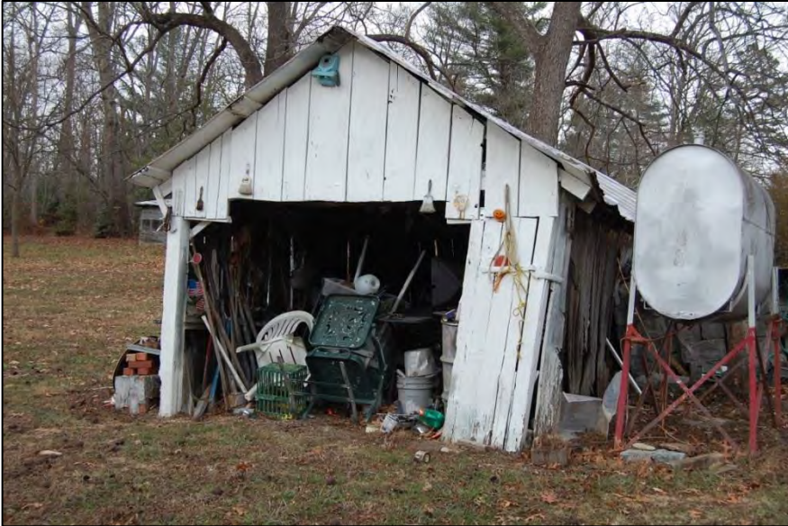
Figure 214. Southwest front and southeast side elevations of garage; chicken coop at left distance
