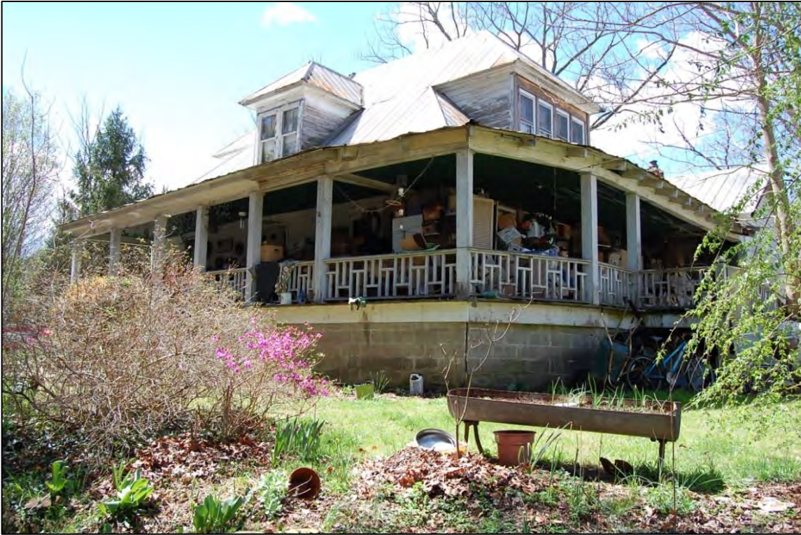
Figure 192. East front and north side elevations; note rafter tails at north-facing section of porch
