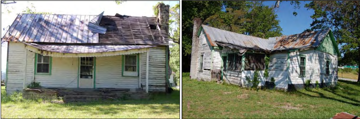
Figure 19. J.J. Justice House (HN-1193): north front elevation, left; east side and west rear elevations, right
