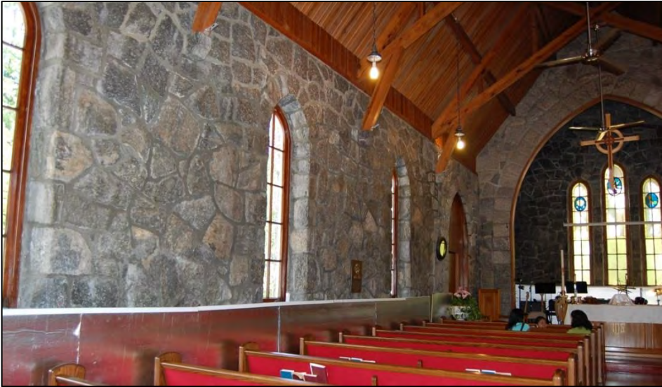
Figure 32. St. Mary's Chapel looking northeast toward chancel; note lightened grout above bays at left (north) from second period of construction and exposed wooden trusses
