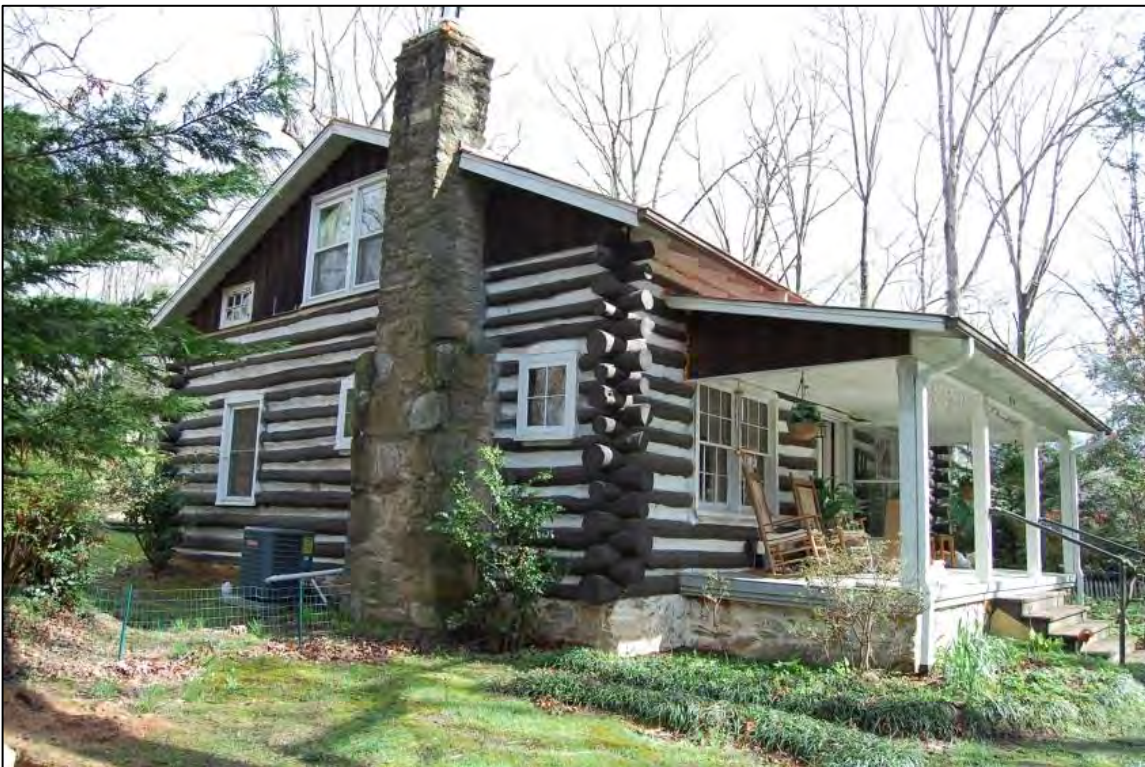
Figure 58. West side and south front elevation of log house; note stone chimney and foundation, thick concrete chinking, and saddle-notching extending well beyond wall planes
